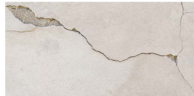
Stress-cracking can be caused by poor embedment or omission of control joints.
