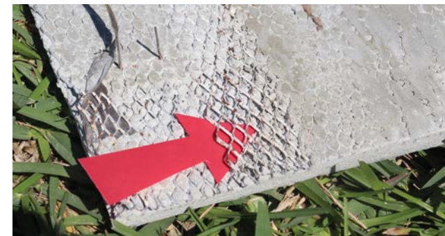
Red arrow shows areas with no embedment, from moisture or corrosion.
